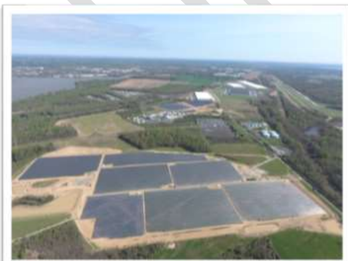
Constellation Energy Perryman Solar Array under construction. Photo provided by Constellation Energy.
